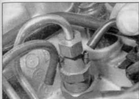
10.5 Pulling a leak-off pipe from a fuel injector
