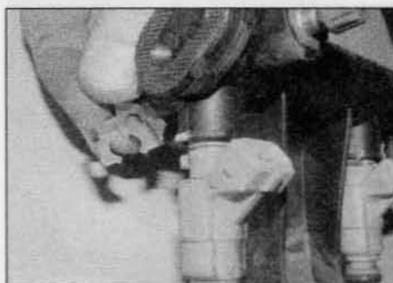
13.15 Slide out the retaining clip(s) and remove the relevant injector(s) from the fuel rail – 1.6 litre models
