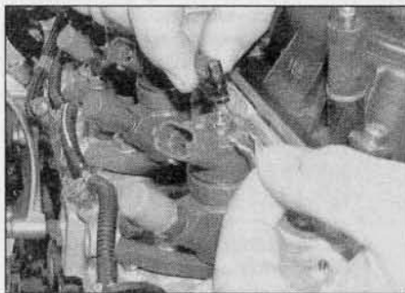
15.15 Remove the retaining clip and disconnect the leak-off pipe connector from the injector – 2.0 litre models
