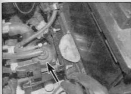
3.32 EGR solenoid valve location (arrowed) on the battery mounting plate – 2.0 litre models
