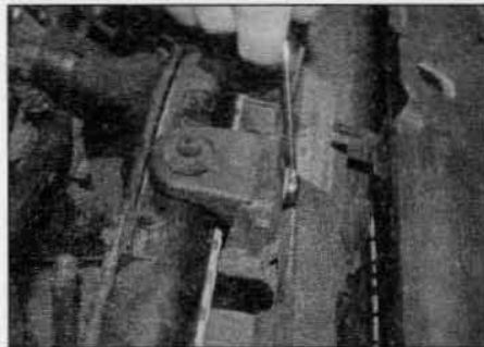
3.22 Undo the bolt securing each radiator upper mounting bracket to the support frame
