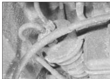
21.1 Fuel accumulator unit location
