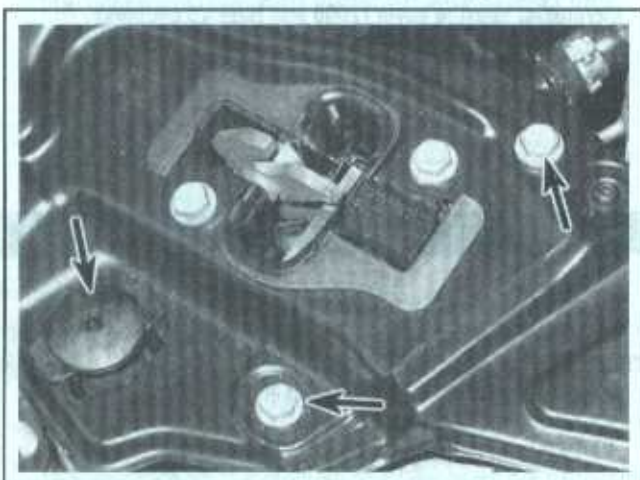
4.13 Unscrew the radiator crossmember bolts and retaining pin from each end of the crossmember
