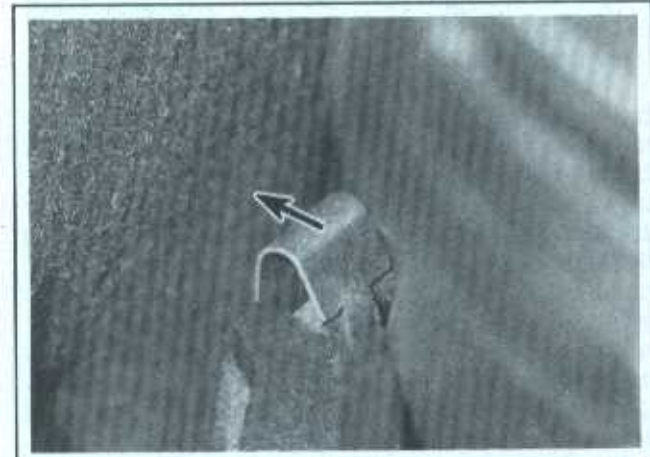
12.5 To disengage the MAF/IAT sensor from the elbow-shaped air intake duct below the sensor, pry this metal spring clamp (on the sensor's lower end, near the firewall) from the sensor with a large screwdriver
