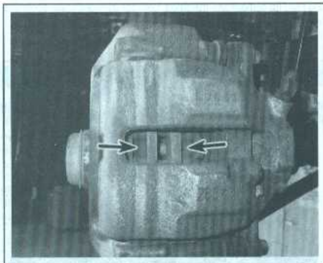
16.7 With the wheel off, check the thickness of the brake pads through the inspection hole (front disc shown, rear disc caliper similar)
