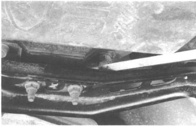
9.2 Pry between the crossmember and the transmission to check for movement of the mount
