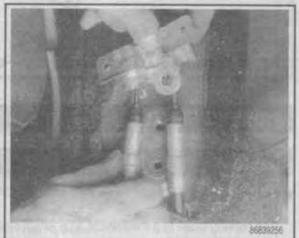
Fig. 83 Free at last: the cables are ready for removal—assuming they are detached at the rear brakes as well
