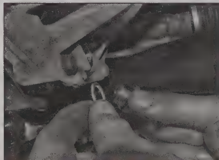
2.7 Fit new sealing washer when refitting
