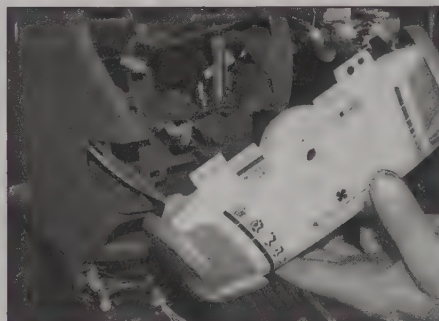
9.7 Note how the air distribution and temperature cables are routed
