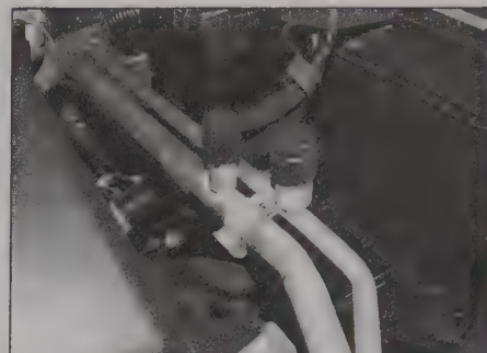
10.2 Air conditioning low- and high-pressure refrigerant pipes
