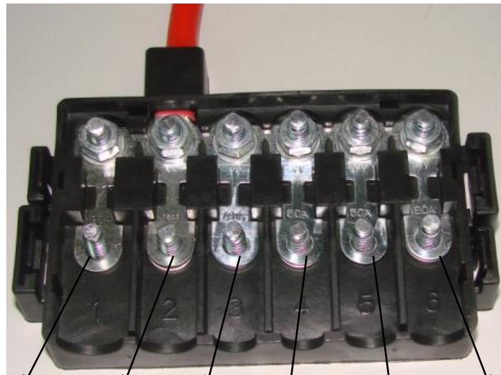
PF1 terminal PF2 terminal PF3 terminal PF4 terminal PF5 terminal PF6 terminal
