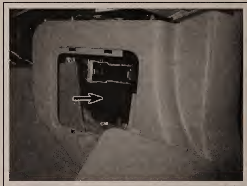
3.1b The other fuse and relay box (the manufacturer calls it the Smart Junction Box) is located inside the vehicle, behind the right kick panel. There's an access door, but it's designed to provide access to the large electrical connector above the fuse box
