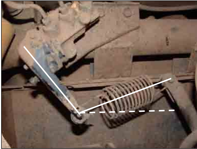
After correction the spring is closer to a 90 degree angle (full line) As opposed to where it was prior to the bracket being fitted (dashed line)
